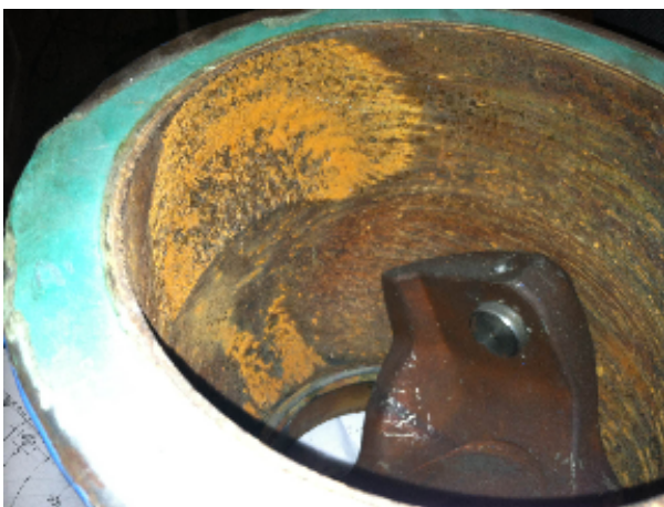
Figure 1. Severe pitting damage from cavitation resulted in a pinhole leak on the valve body of a V-notch Ball Valve used to regulate the cooling water flow to aluminum casting molds.
